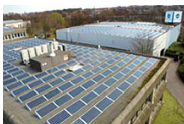
Photovoltaic installation on the roof of the company building (Belgium)
